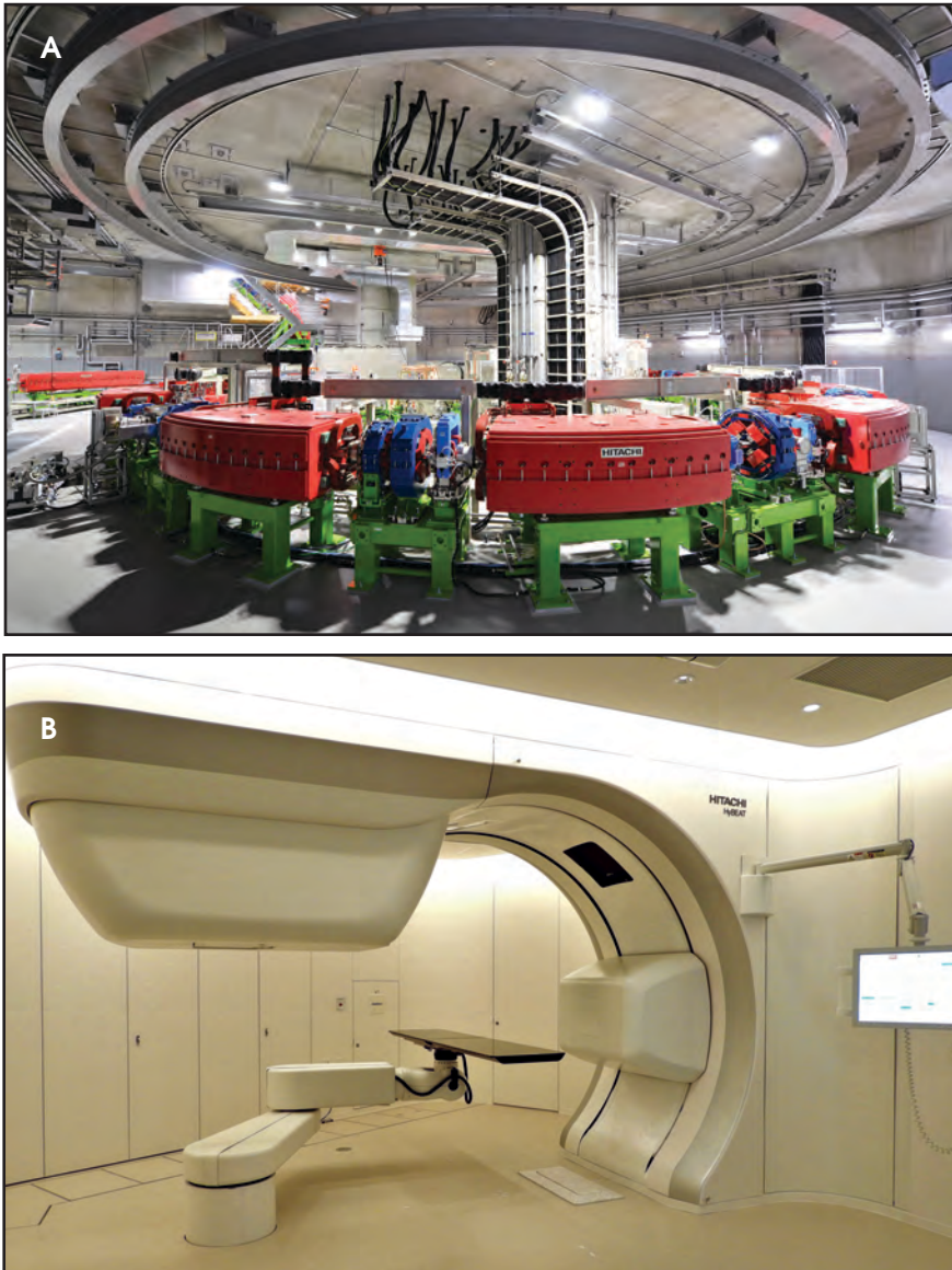
FIGURE 1. An accelerator room at the Osaka Heavy Ion Therapy Center (A). Example of a treatment room at the center (B). photos courtesy Hitachi Ltd.
