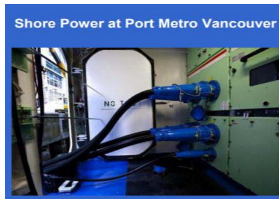
Figure 4: Shore power services at Port of Metro Vancouver (The Port of Metro Vancouver, 2017)
