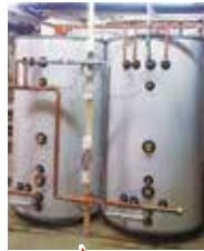
Hot water tank (2qty)
