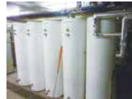
Hot water tank 400 L×10
