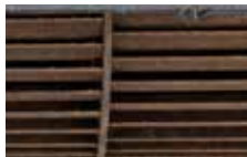
No Dual Barrier Coating Used
